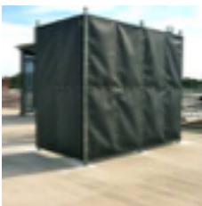
Figure 16: Environmental controls; cut zone filter screens
